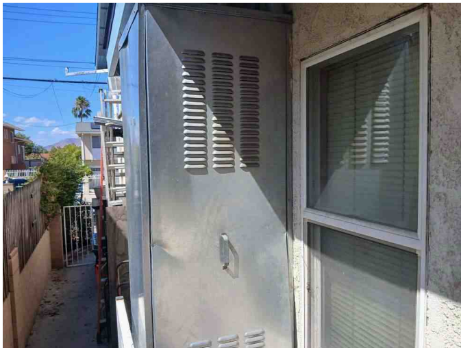
Please note that water heater was not accessible due it being enclosed and bolted in.
