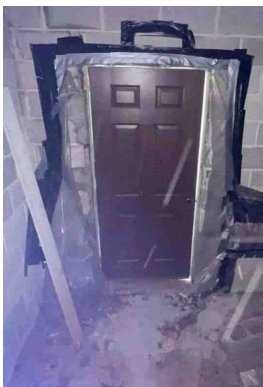
Repair door/trim out properly
