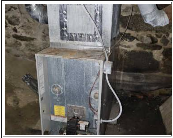
Forced hot air heating system
