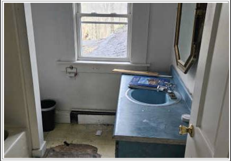
Comment: Bathroom Unit 3
