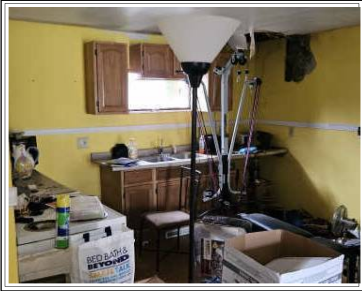
Second view kitchen Unit 4--water damage ceiling
