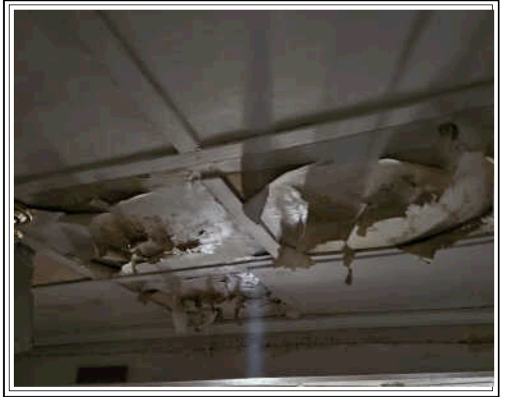
Water damage ceiling Unit 1
