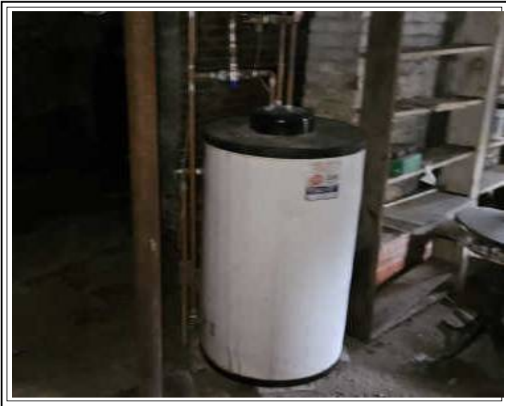
Hot water heater
