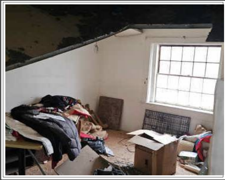
Ceiling falling in Unit 4 living room
