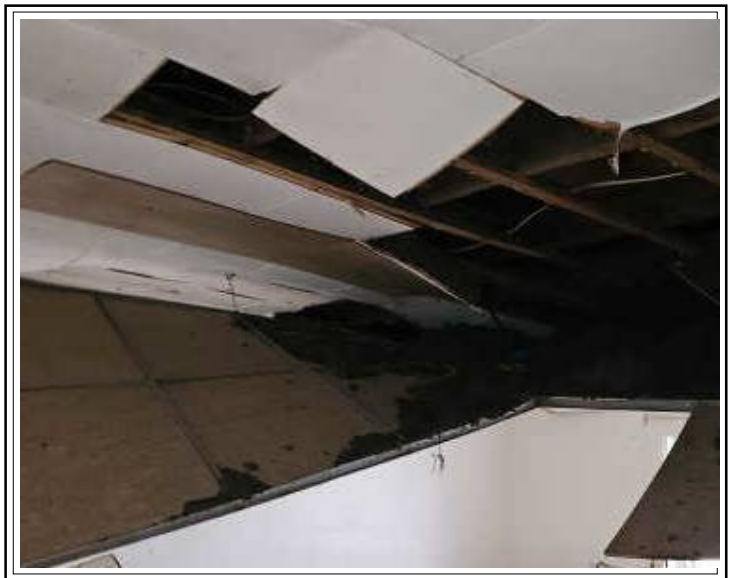
Ceiling fell in Unit 4
