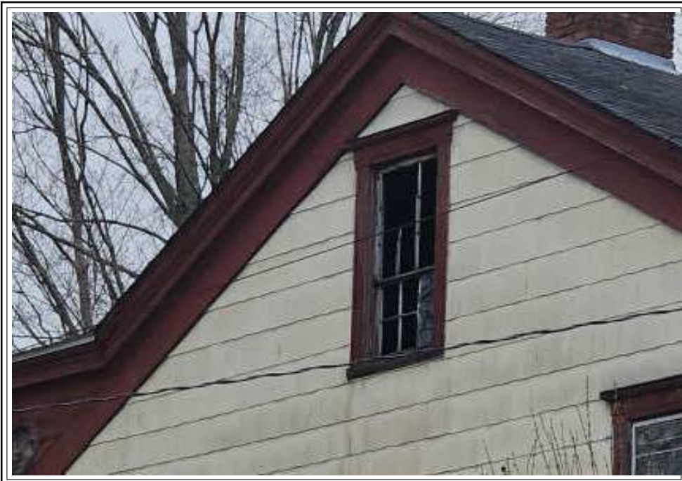
Broken attic window
