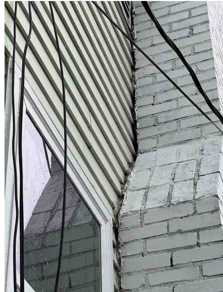
There appears to be progressive separation from chimney and dwelling.
