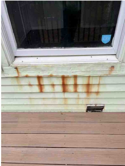
Moisture damage under window seal. Recommend a general contractor view/access/correct as needed
