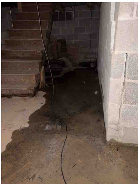
Seperation of block and moisture in basement & crawl area
