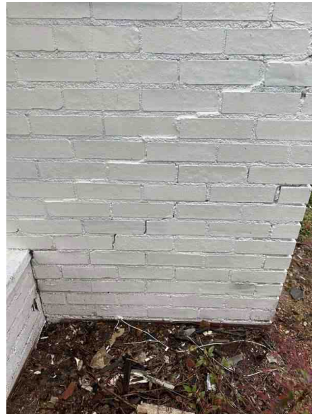
Appears to be settlement on exterior brick
