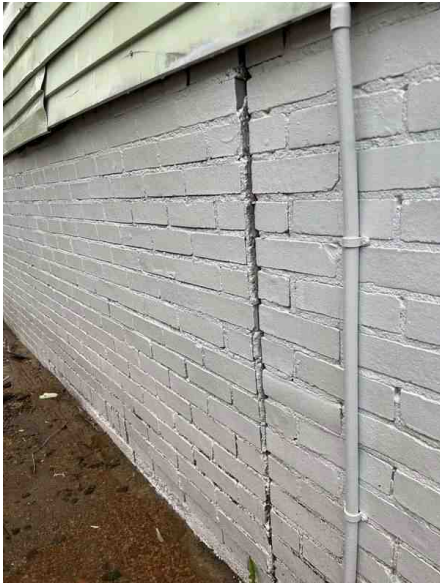
settlement crack appears significant in size. Nearly 1 full inch
