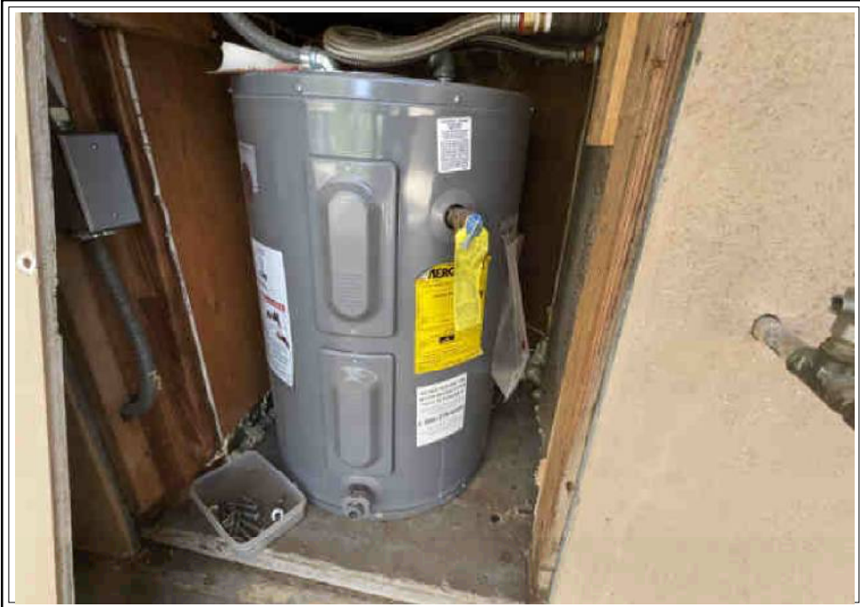
Hotwater Heater w/o Seismic Straps
