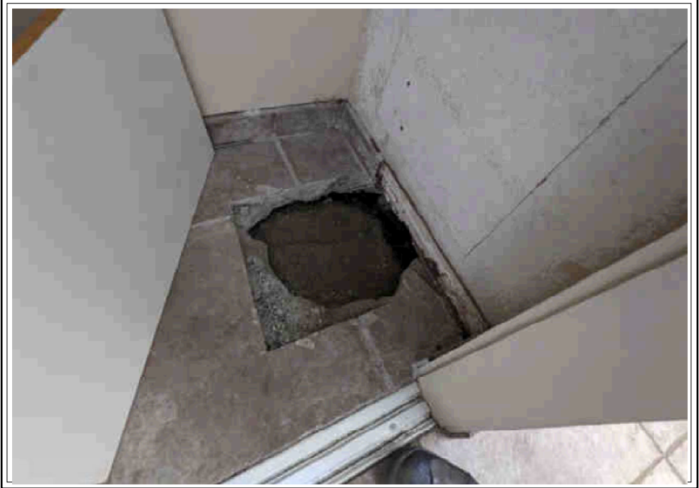
1st bedroom floor damage.
