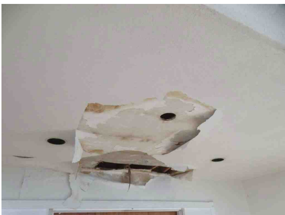
Living Room Ceiling Water Damage
