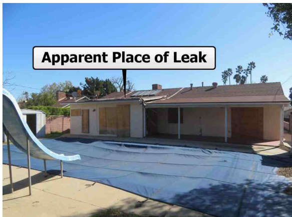
Exterior Photo Focusing on Roof Leak
