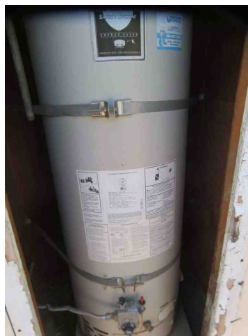
Double Strapped Water Heater
