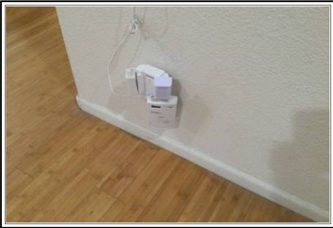
Carbon Monoxide Detector on the Second Floor
