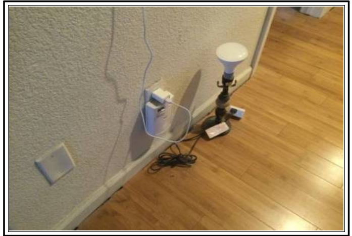
Carbon Monoxide Detector on the Third Floor
