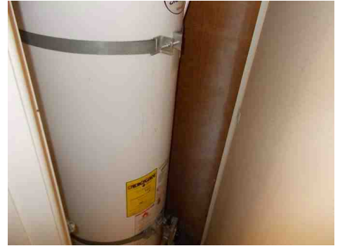
Water heater w/straps
