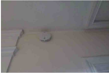
Carbon / Smoke Detector
