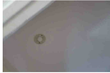
Rear Unit Missing Smoke Detector
