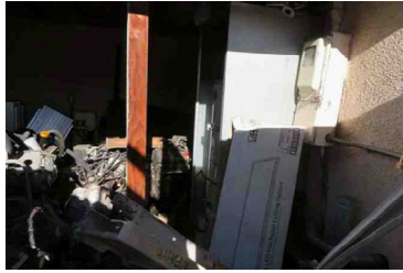
Rear Unit Missing Smoke Detector
