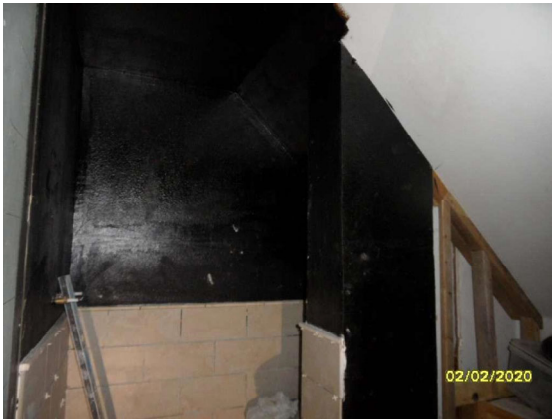
Room #3 Requires completion
