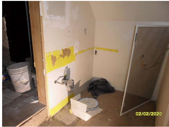
Room #3 Requires completion
