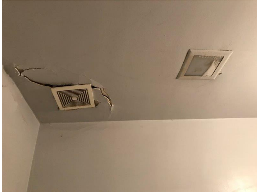
View of Deferred Maintenance
