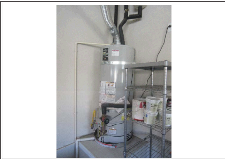
Hot water heater
