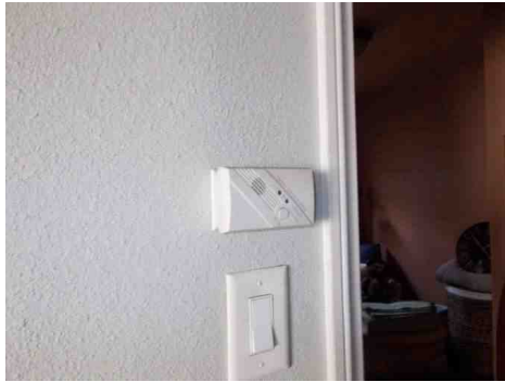
Subject CO Alarm
