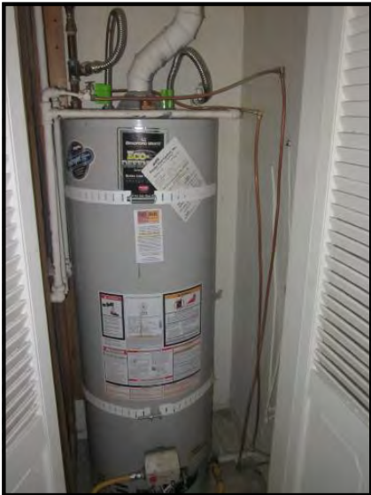
Unit 1 Water Heater
