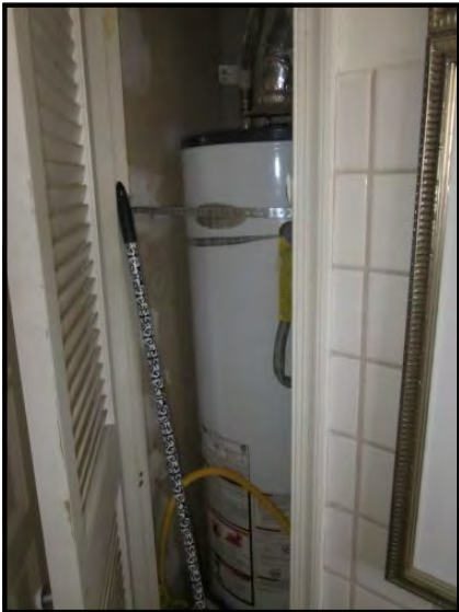
Unit 2 Water Heater
