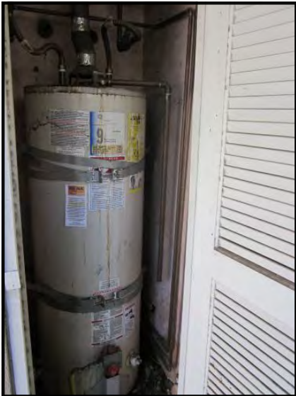
Unit 3 Water Heater
